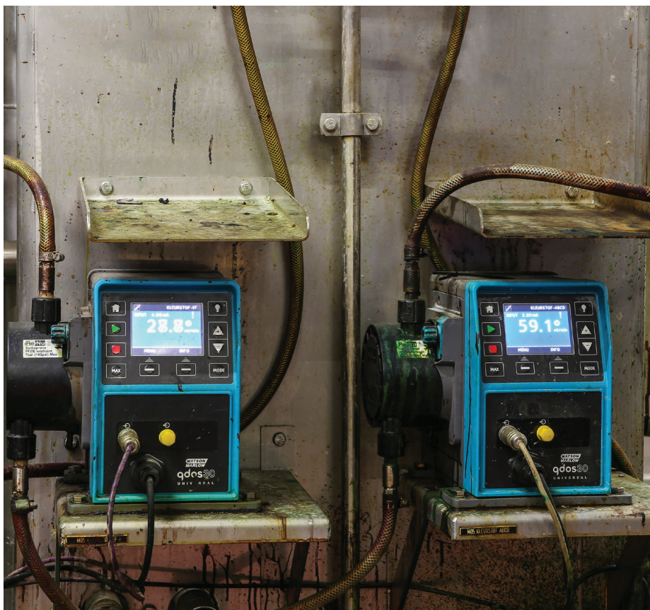
Above: Qdos pumps used for colourant dosing
