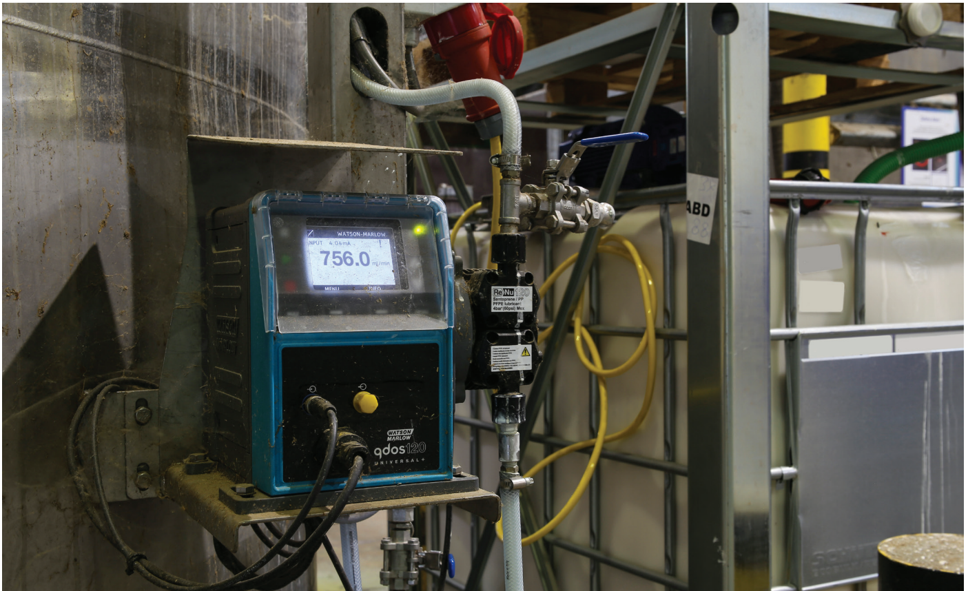
Above: A Qdos 120 pump used for dosing lime slurry
